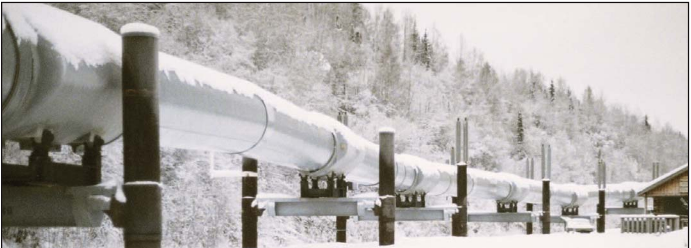
The 800 mile long 48 inch diameter Trans Alaska Pipeline System was constructed using Lincoln Electric Pipeliners® welders.
